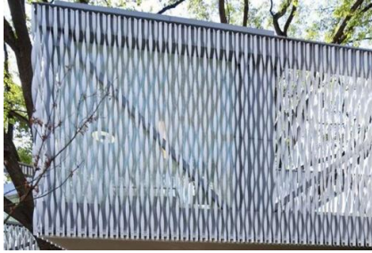
Fig. 12. Element's Distortion: Twisted Elements - Huaxin Business Center, in Xuhui, China.
