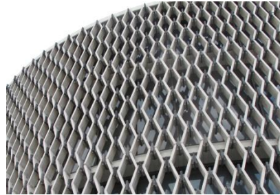
Fig. 15. Element's Distortion: Bended Elements - Pan American Health Organization Building, Washington DC , USA.
