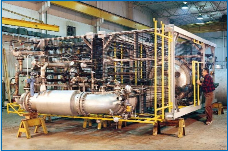
Figure 20. Typical high vacuum distillation system under final shop assembly.
