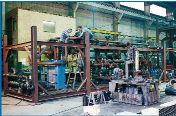
Figure 19. Here the condenser, decanter and heat exchangers were assembled in the shop on three horizontal modules.
