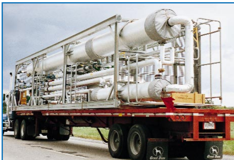
Figure 17. Modular distillation system during transportation.
