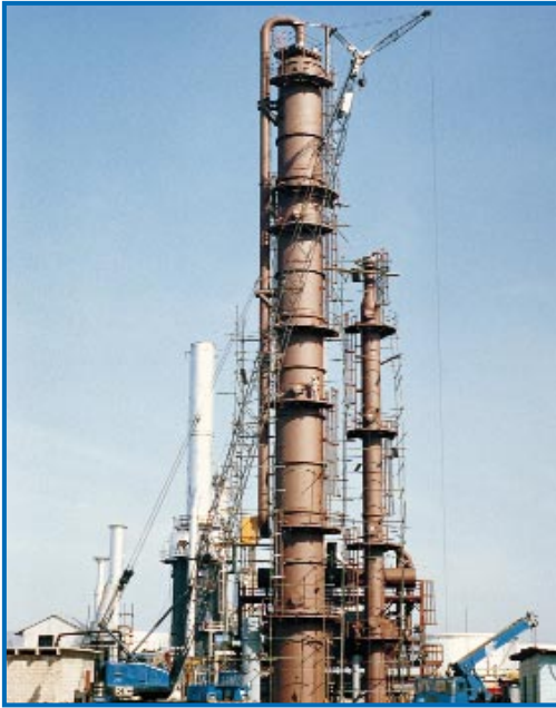
Figure 18. Petrojam where the 10 ft (3m) diameter column and reboiler are self standing.
