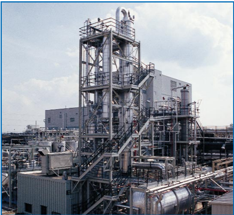
Figure 13. Batch distillation system.
