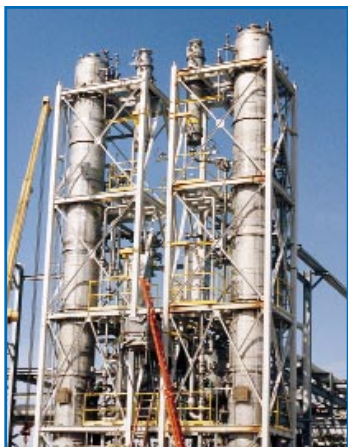
Figure 10. Two steam strippers.
