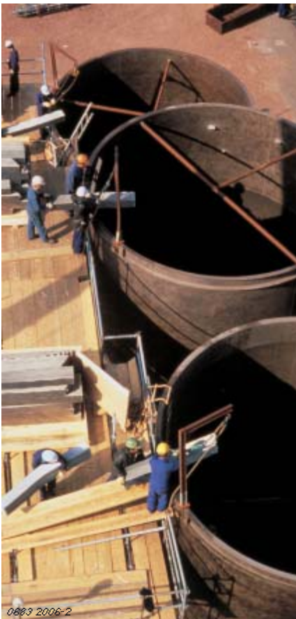
0683 2006-2 The packing is fitted inside the column sleeves at the preassembly site
