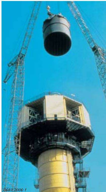
0683 2006-1 The column sleeve is lowered into the column with two cranes. Weight: 100 tons
